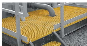
Raised work platforms
