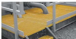
Raised work platforms
